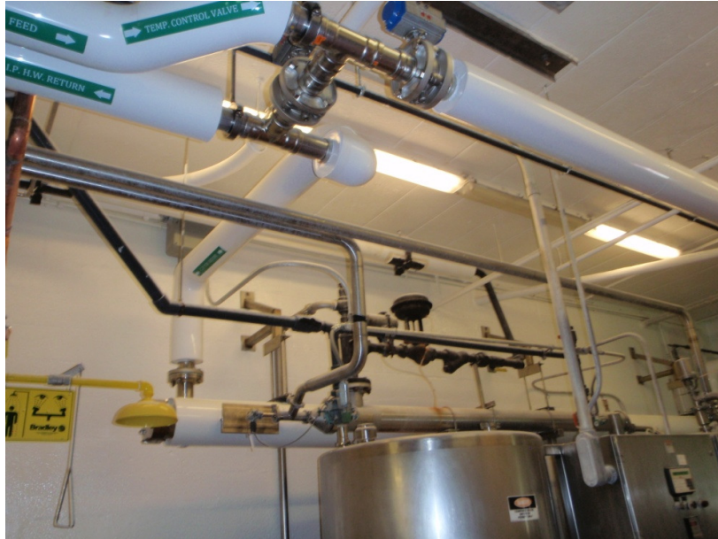
SS Sanitary Piping from the Batter CIP Pump to new Batter Heat Exchanger
