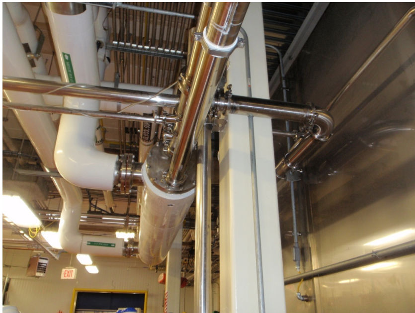
Freezer CIP Heat Exchanger and SS Sanitary Piping
